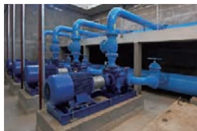
Building water pumps
