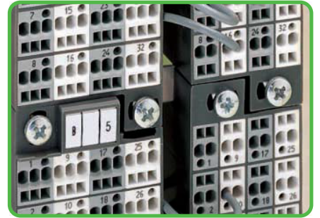
Slimline matrix patchboard (lower right), mounted upside down.
