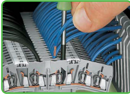
Terminal blocks for matrix patching. Conductor termination/removal in center of the terminal block.
