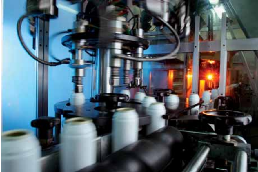
Can filling plant controlled by Mitsubishi GOTs
