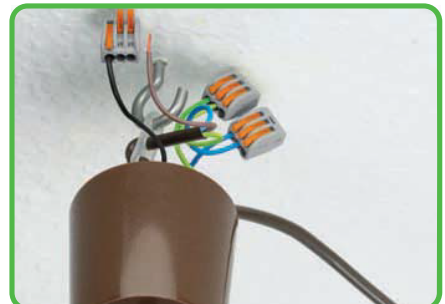
Lighting fixture connected with flexible power feed.
