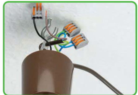
Lighting fixture connected with flexible power feed.
